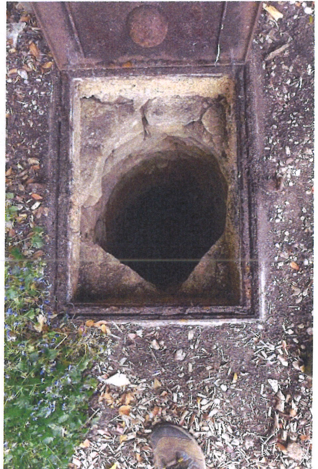
D-16 Well-head at 2 Dynevor Place
