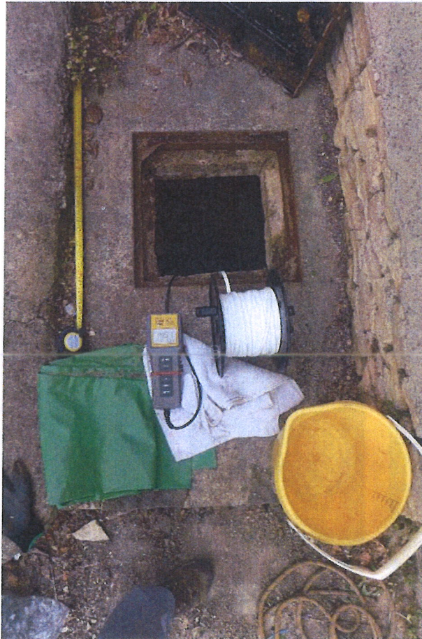
D-15 Well-head at Coln House West
